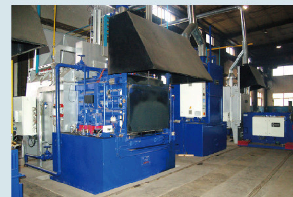
Germany Ipsen controlled atmosphere furnace heat treatment production line
